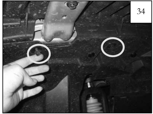
Reinstall two factory bolts as shown as well as reinstall marker light wiring.
